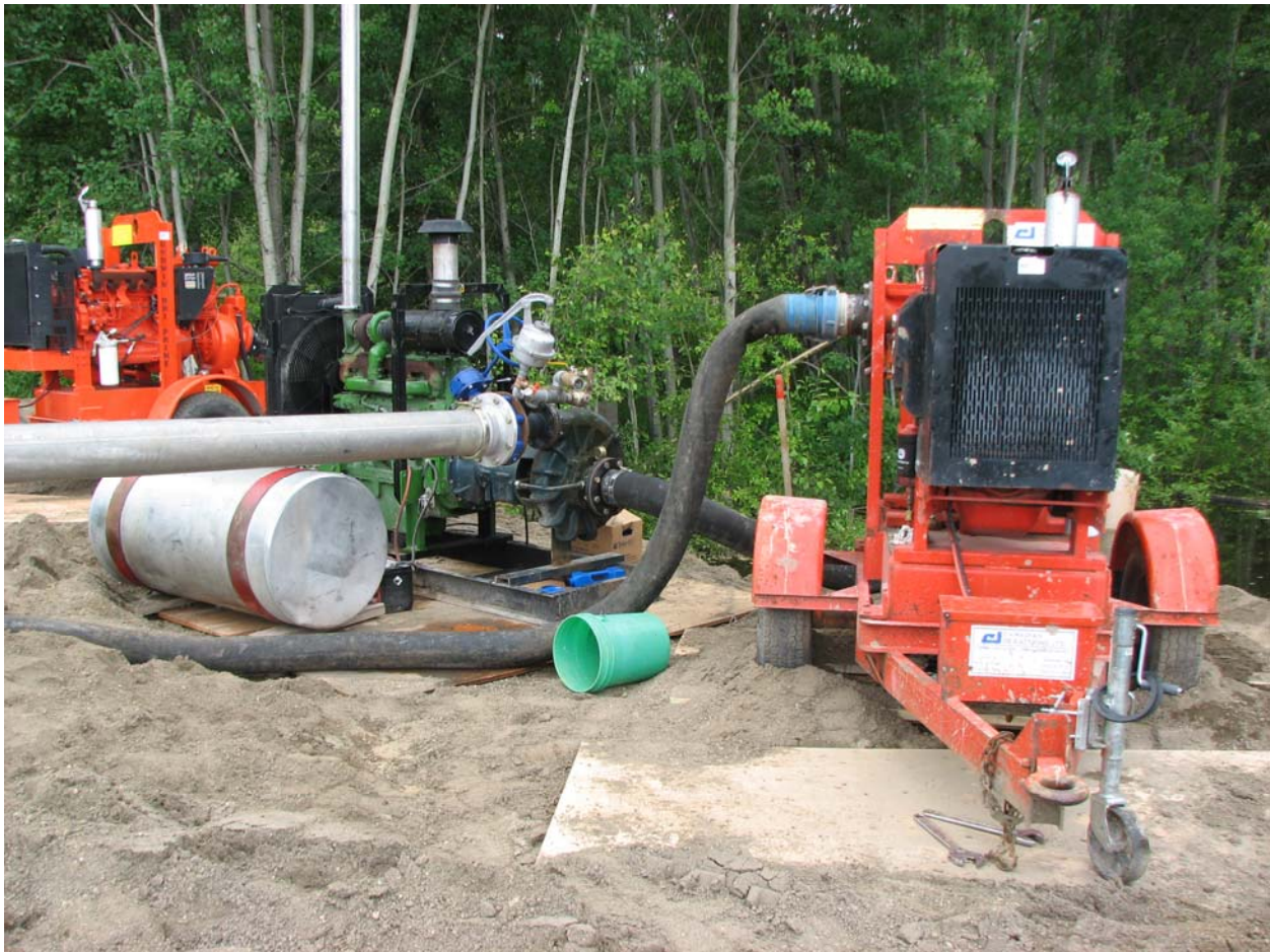
Figure 2 – Temporary Mobile Pump Station
